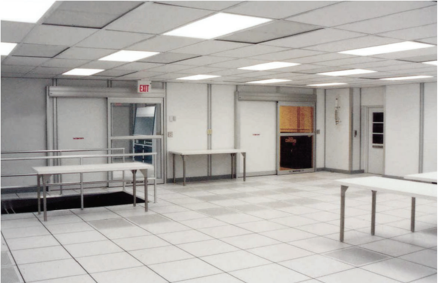
Class 100 (ISO 5) Cleanroom with Raised Floor (at rest).
